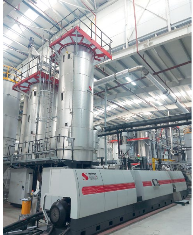
Starlinger's recoSTAR PET 215 iV+ bottle-to-bottle recycling line installed at Tanrikulu's Akyazi plant in Sakarya Province, Türkiye, produces 2.4 tons of food-grade rPET pellets per hour (©Starlinger)
